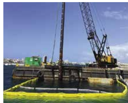
Nucor Skyline spiralweld pipe piles being driven to repair Pier 3 in Old San Juan, Puerto Rico.
